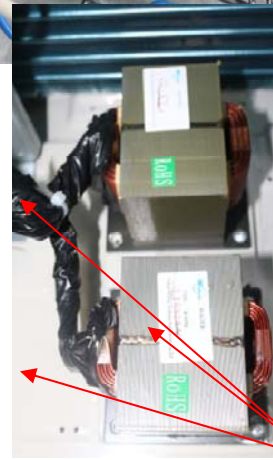
Screws of reactor
