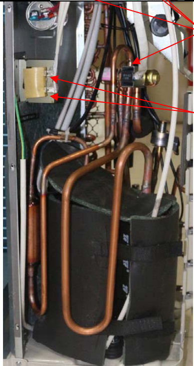
Screws of reactor
