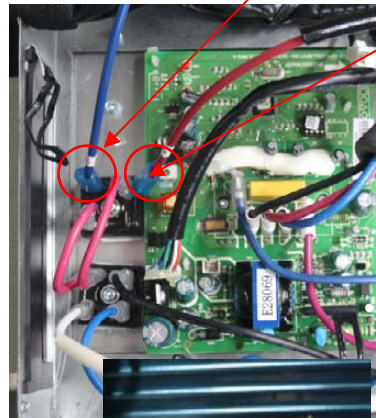
Connection wirings of reactor2 (red, red)
